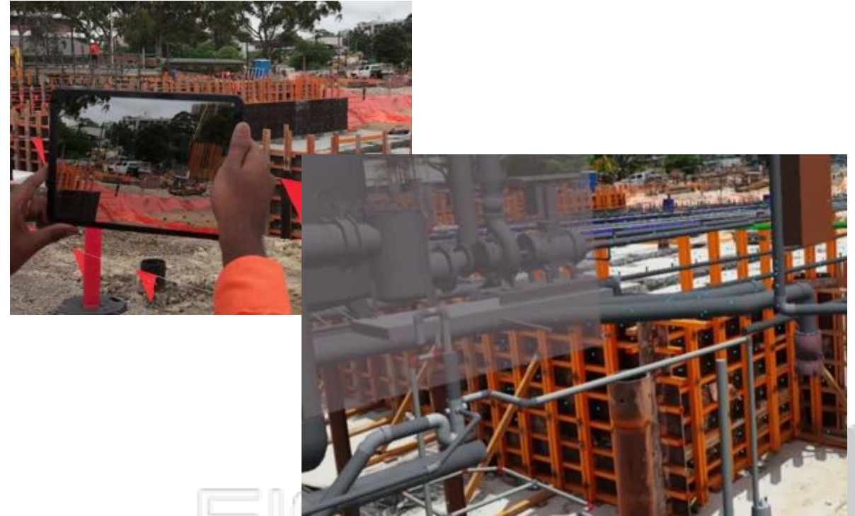
Gunyama Park Aquatic and Recreation Centre – CPB Contractors Client: City of Sydney
